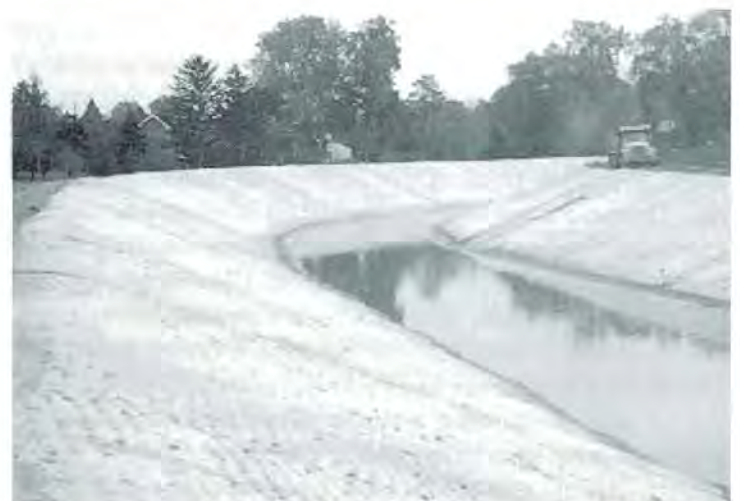
Realigned, Fabriform®-paved Euclid Creek, looking upstream. Truck on right bank is delivering fill for finish grading berms.
