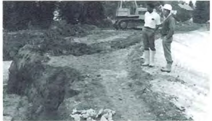
During the period of Fabriform placement, heavy rains often posed problems. Here, a temporary diversion ditch was overtaxed to the point of nearly undermining a newly-installed section of Fabriform.
